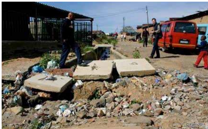
Illustration 3: A dilapidated storm water drain in Tembisa, full of litter and poorly-maintained (but only 6 months old). (Photograph courtesy of Christina Fatti).
